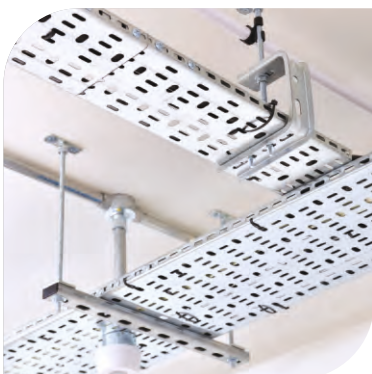
CABLE TRAY, ANCHORS AND FASTENERS
